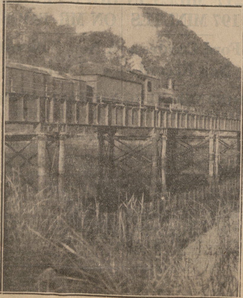
SCENE OF RAILWAY WASHAWAYS.—The Fairy Knowe Bridge on the George—Knysna line, the piers of which have tilted as the result of the New Year washaways.
