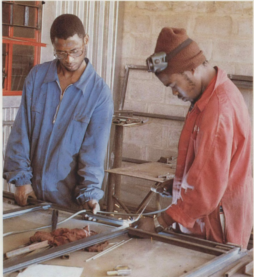
Self-help housing encourages township production of building materials, such as metal window frames at Katlehong, near Germiston on the East Rand
