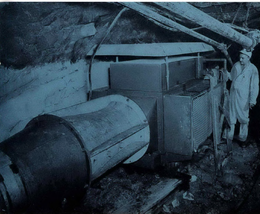
A portable refrigeration unit, used for cooling underground workings at Western Deep Levels
