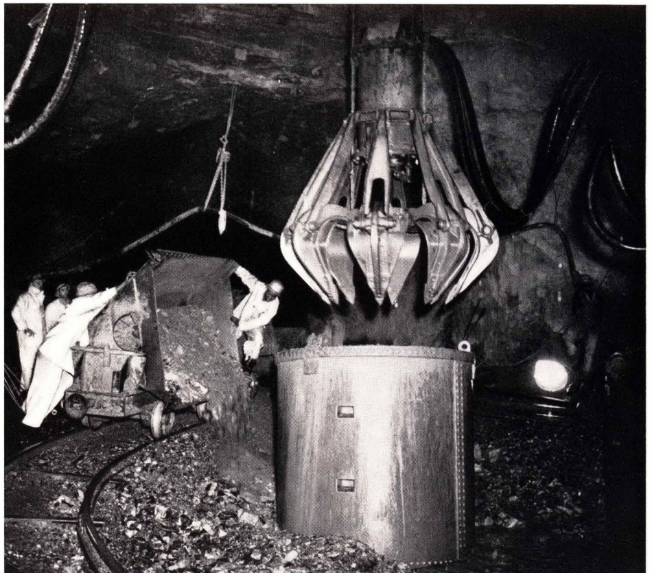
A pneumatically operated cactus-type grab drops broken rock into a kibble for hoisting to the surface during shaft sinking and station cutting at the Western Holdings mine
