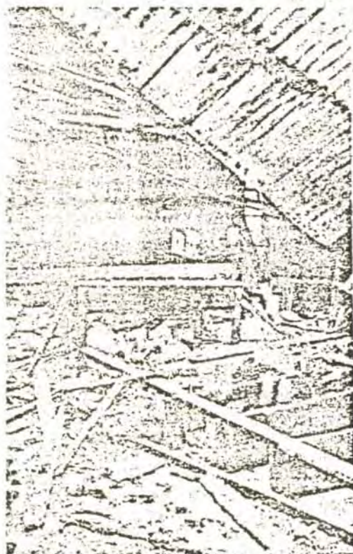
The gutted interior of the Moroko police station in Soweto after Umkhonto we Sizwe guerrillas had carried out a highly successful attack in May of this year.
