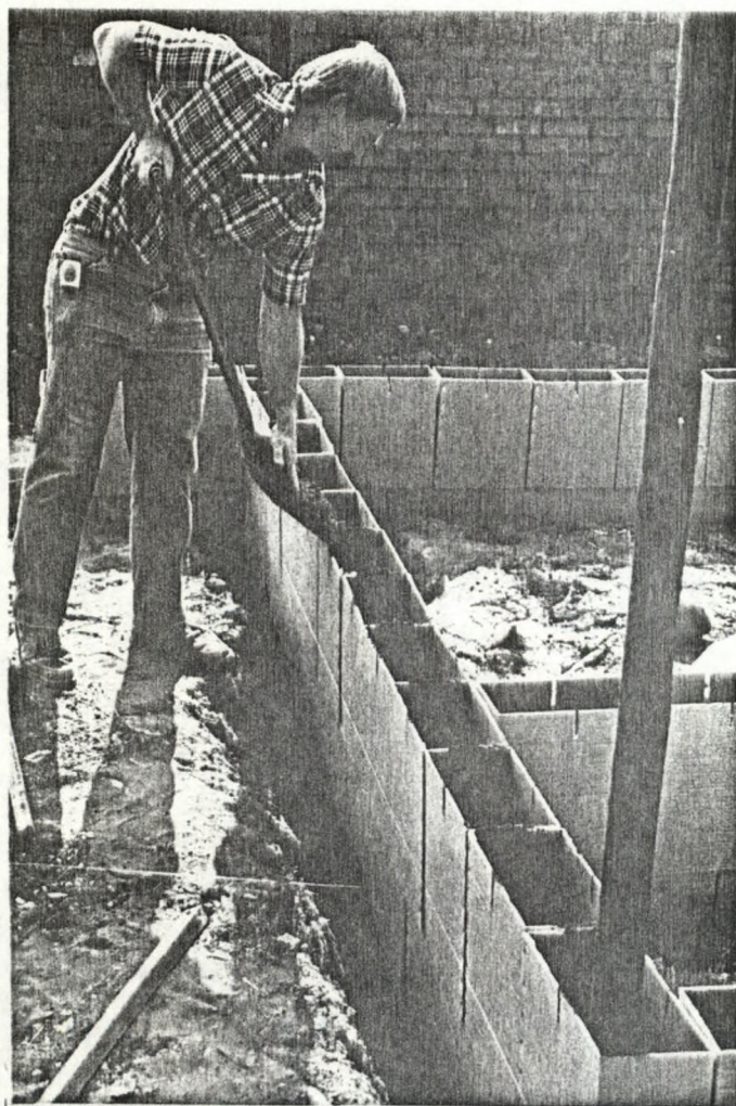
FIRST COURSE FILLED WHILE SLEEVE LOCATED BY SECOND COURSE, ie. LAY TWO FILL ONE.
