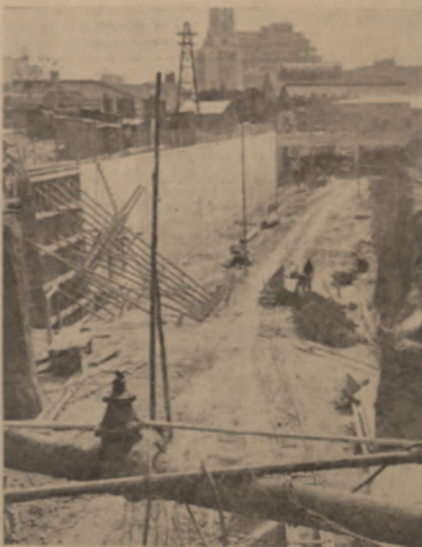
A new station for the increasing traffic from Orlando and adjoining townships is to be built at the corner of Faraday and Eloff Streets. The photograph shows the site of the platforms in the foreground. An underground extension from the present Village Main station, off Eloff Street Extension, will link up with the new terminus.
