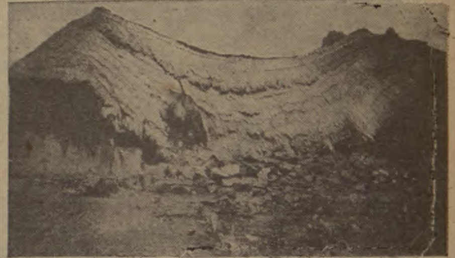
Without warning, this school building collapsed on a Wednesday morning. It was a fine, clear day. At the time, there were 93 children and the principal, Mr. Stephen I. P. Kgame, in the class-room. By a miracle, nobody was hurt. It is the Schaumburg Community School at Die Moot in the Krugersdorp District.
