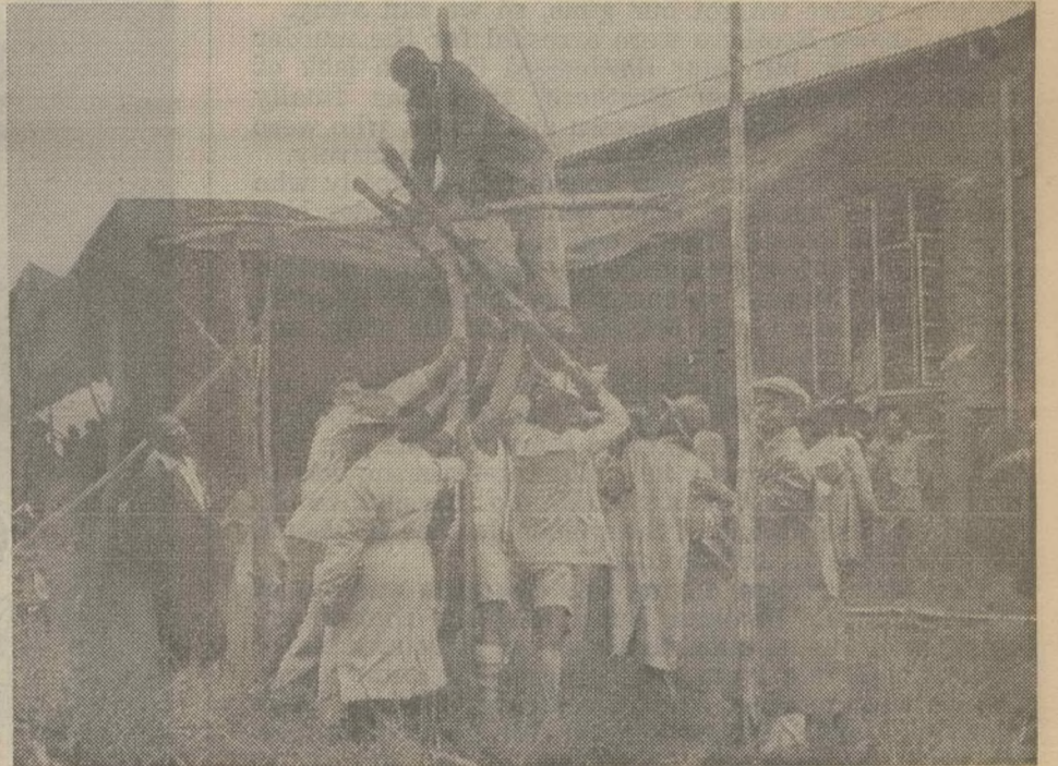
DELEGATES PLAY BUILDER The hall is packed to capacity. Many can't get in. Shelters are put up hastily to protect them from the rain.
